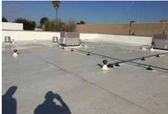
Typical roof and AC units at M&O building
