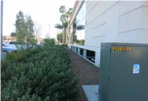
East side of building; transformer
