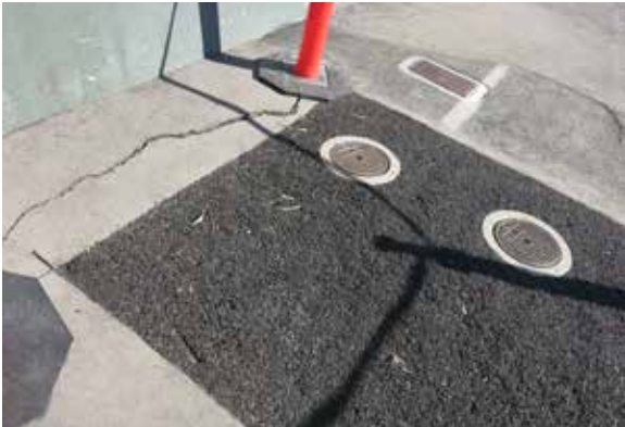
Paving cracking and patching throughout paved areas of the site
