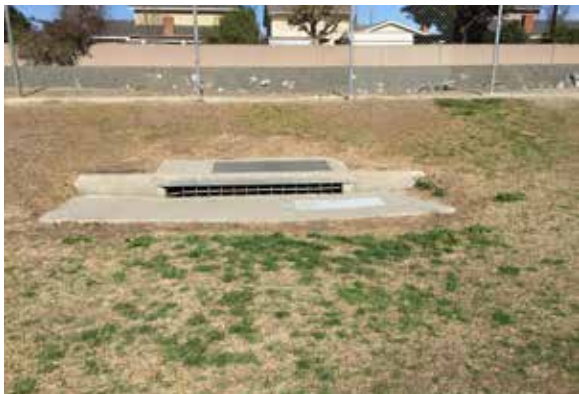
Playfield drainage system
