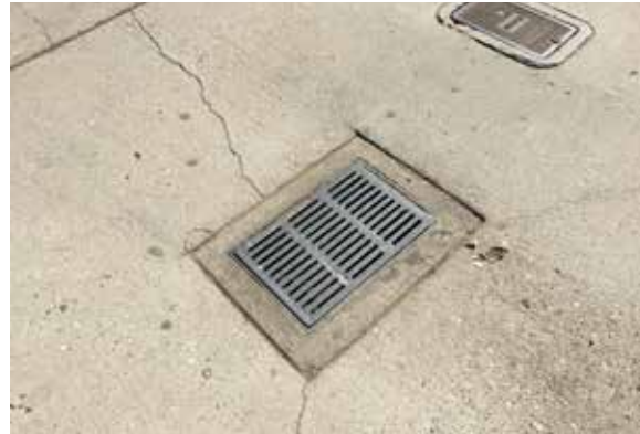
Exterior area drains; cracks in paving
