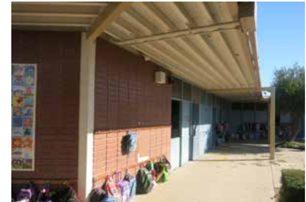
Typical exterior of building: covered walkway, backpack hooks, door and window system
