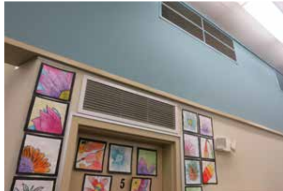
Vents for air circulation for whole building exhaust system
